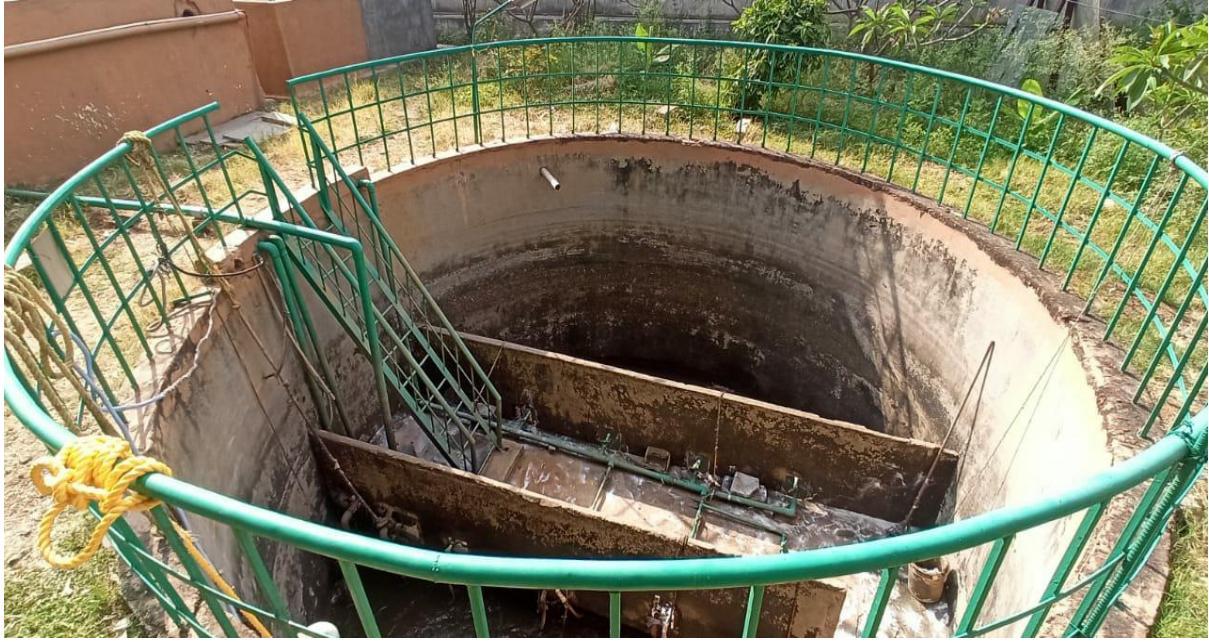
Recycling of waste water
